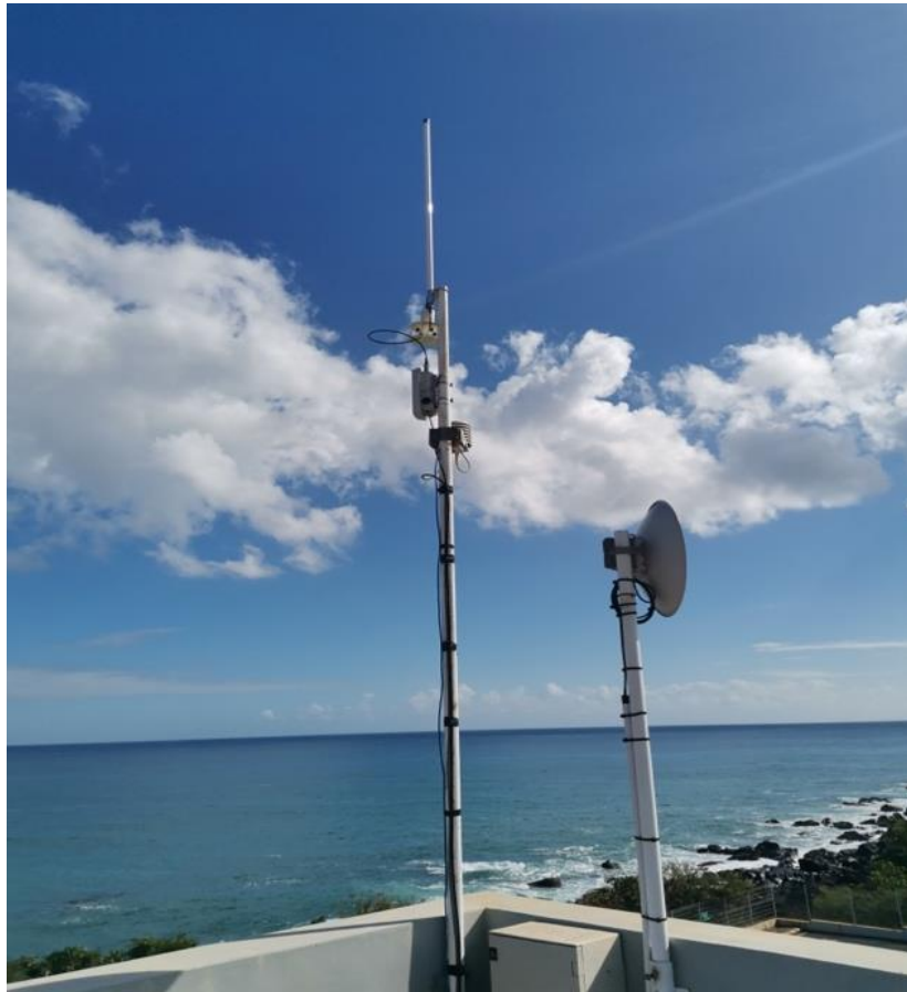
Kerlink Wirnet iStation deployed in Albion Source: Digital Twin Services ©2022
