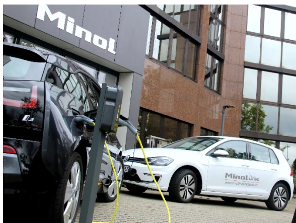
Picture Caption: All signs point to e-mobility: charging stations will be part of the standard appointments of real estate properties in future. Source: Minol-ZENNER
