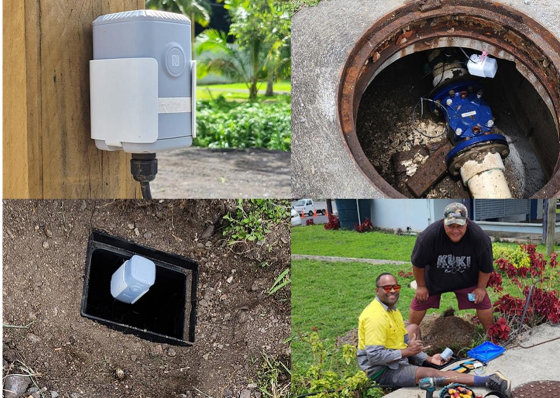
On-site deployment of Milesight sensors
